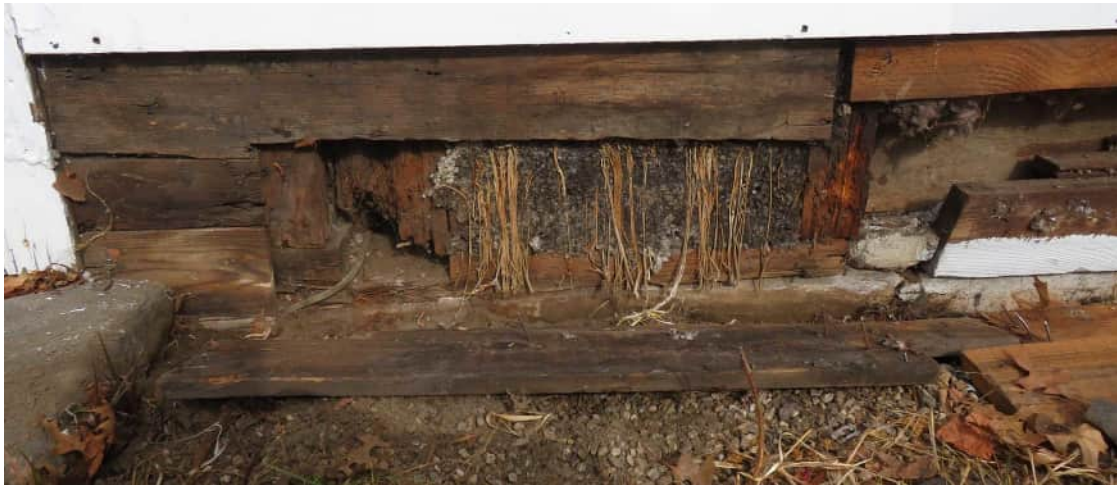
Deteriorated portion of the south sill and post
