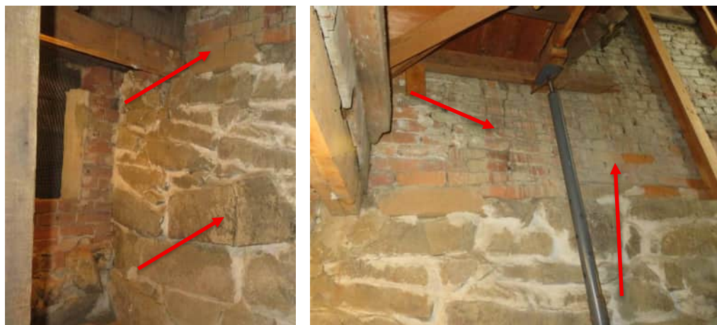
South wall of chimney base, red arrows indicate cracks and water staining
