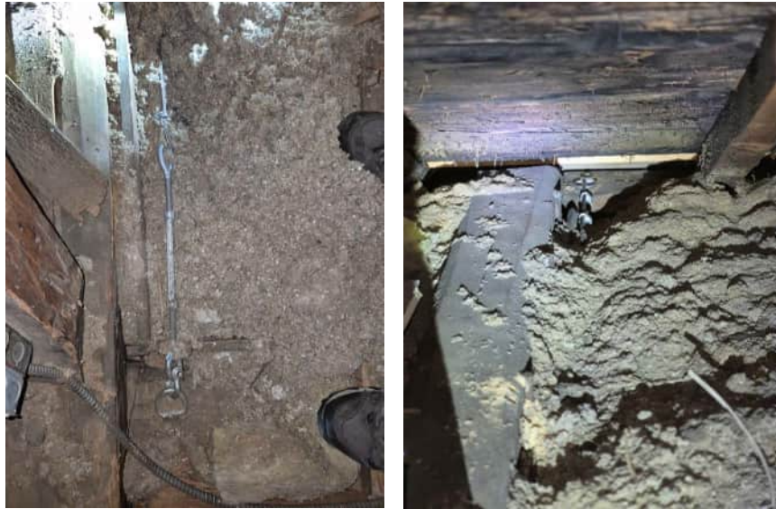
Cable ties over lean-to in attic
