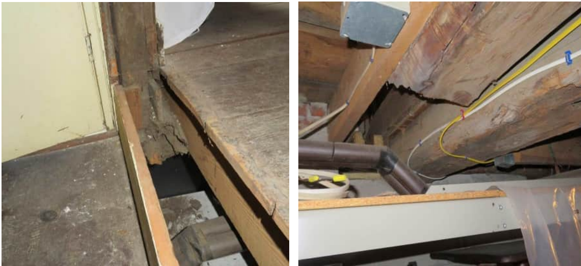
Top: Looking down at door threshold without trim; Bottom Left: Looking east to end of abandoned timber; Bottom Right: Looking west at augmented framing from below.
