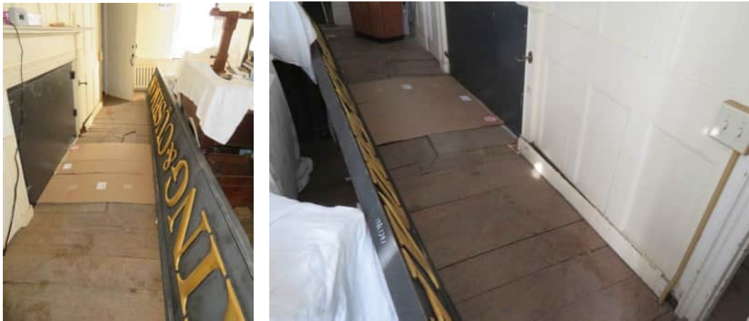
Deflection at hearth in west room, from north and south respectively
