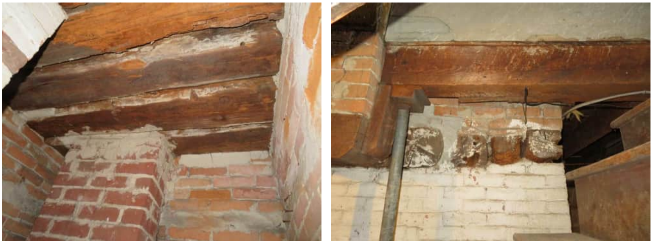
Deteriorated timber platform supporting Kitchen Ell chimney mass above
