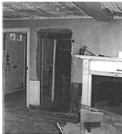
Figure 79. Left – Drawing of the Phase 4 chimney breast wall in Rm 102 after the cellar stairs were relocated to the southwest corner of Rm 110 during the Phase 4 remodeling. At that time the former door opening was lathed and plastered. Note the settling in the floor from left to right in both the drawing and photograph as indicated by the level of the ceiling and the fireplace mantelpiece. (Drawing from Clancey and Leeke, 1992.)
