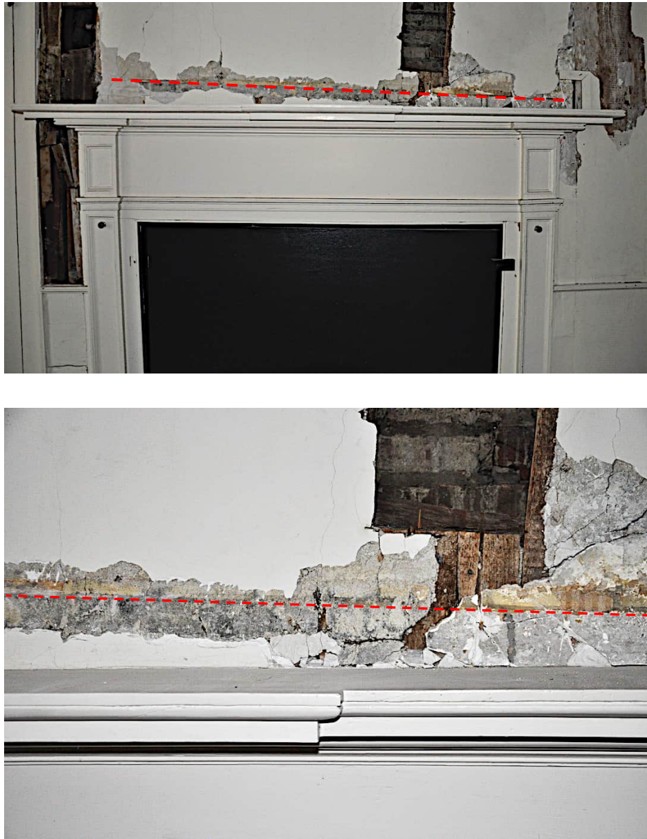
Figure 82. Top – View of the expanded excavation through the plaster above the mantelpiece in Rm 102 undertaken to reveal the full extent of the overmantel decorative painting. The red dashed line indicates the degree of settling which occurred since the early-mid 19 th century due to the deterioration of the north sill of the house. The mantelpiece had settled with the walls and floor, but during the 1981 renovations, which included leveling the floor in this room, the mantelpiece was removed and reapplied over the newly-leveled floor and fireplace hearth.
