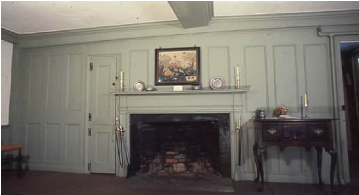
Figure 56. View of the east wall of the parlor, late 20 th century. By the time the paneled chimney breast wall was constructed in the early 19 th century the rear (north) sill had suffered significant deterioration as illustrated by the narrowing space between the top of the panels and the bottom of the girt. The paneled chimney breast wall was clearly built to the already settled north wall and cased chimney girt, but no effort was made at that time in the early 19 th century to raise and level up the frame of the house. (Courtesy of Historic Northampton Archive.)
