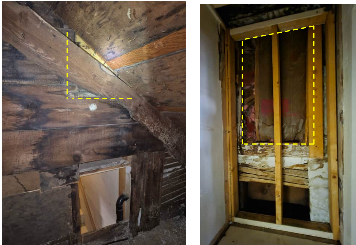
Figure 61. Left – View of the north wall of the Phase 3 raised second-story of the rear pile of the house from the garret of the Phase 5 one-story rear kitchen ell. They yellow dashed lines indicate the location and remains of the window opening and window trim. The opening below the former window is a modern access port to the rear ell garret.
