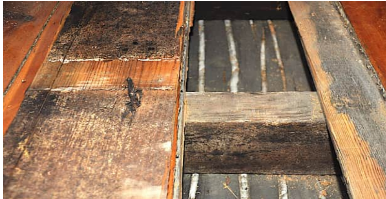
Figure 10. View of the floor joist and underside of a floorboard (on the left) in the ceiling of the hall (Rm 102). Note the dark soot/smoke/grease staining on the sides of the joist and on the floorboard, in contrast to the portion of the floorboard which lay over the joist. Note also the traces of whitewash. (Photograph by Myron O. Stachiw, 2024.)
