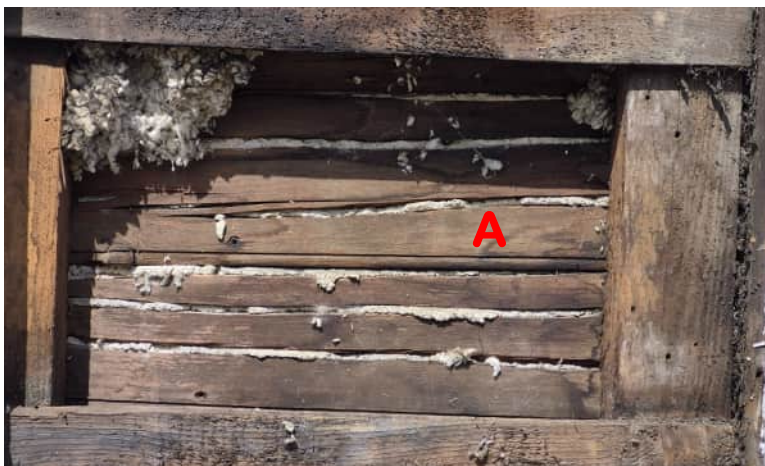
Figure 50. View of the exterior south wall of the west parlor between the two existing windows. Removal of an exterior siding board revealed former exterior door- or window trim (A) reused as split lath. Note that the board was planed smooth and a bead had been applied on one edge. (Photograph by Myron O. Stachiw, 2025)
