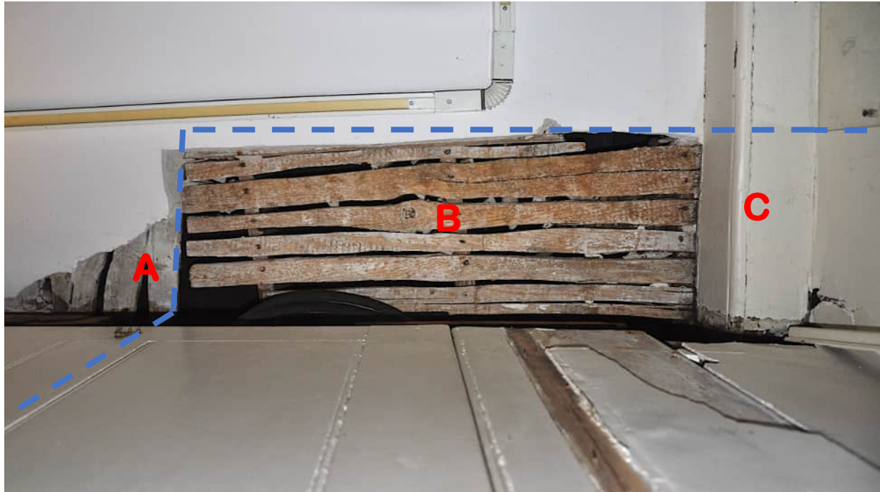
Figure 39. View of the hall/kitchen ceiling in the northwest corner of the room against the west (bottom) and north (right) walls of the room. Plaster has been removed to reveal a patch B in the original ceiling lath A . Note the original Phase 2 ceiling lath A was applied to joists in the ceiling in an east-west orientation, as the joists are oriented north-south. Lath B was applied in a north-south orientation to nailers introduced between the existing joists. The lath A was applied against the east and south sides of the cupboard (blue dashed lines indicates the outline of the cupboard). C is the cased girt on the north wall of the room. The cupboard was removed during the second Federal Period remodeling during Phase 4, which involved a major reconfiguration of the chimney breast wall of this room. This included a partial dismantling and blocking of the bake oven; reduction of the size of the firebox; partial dismantling of the Phase 2 paneled chimney breast wall; erection of a new wall several inches in front of the former paneled wall; construction of a new wall cupboard in front of the former bake oven; and installation of a new mantelpiece. (Photograph by Myron O. Stachiw, 2024.)
