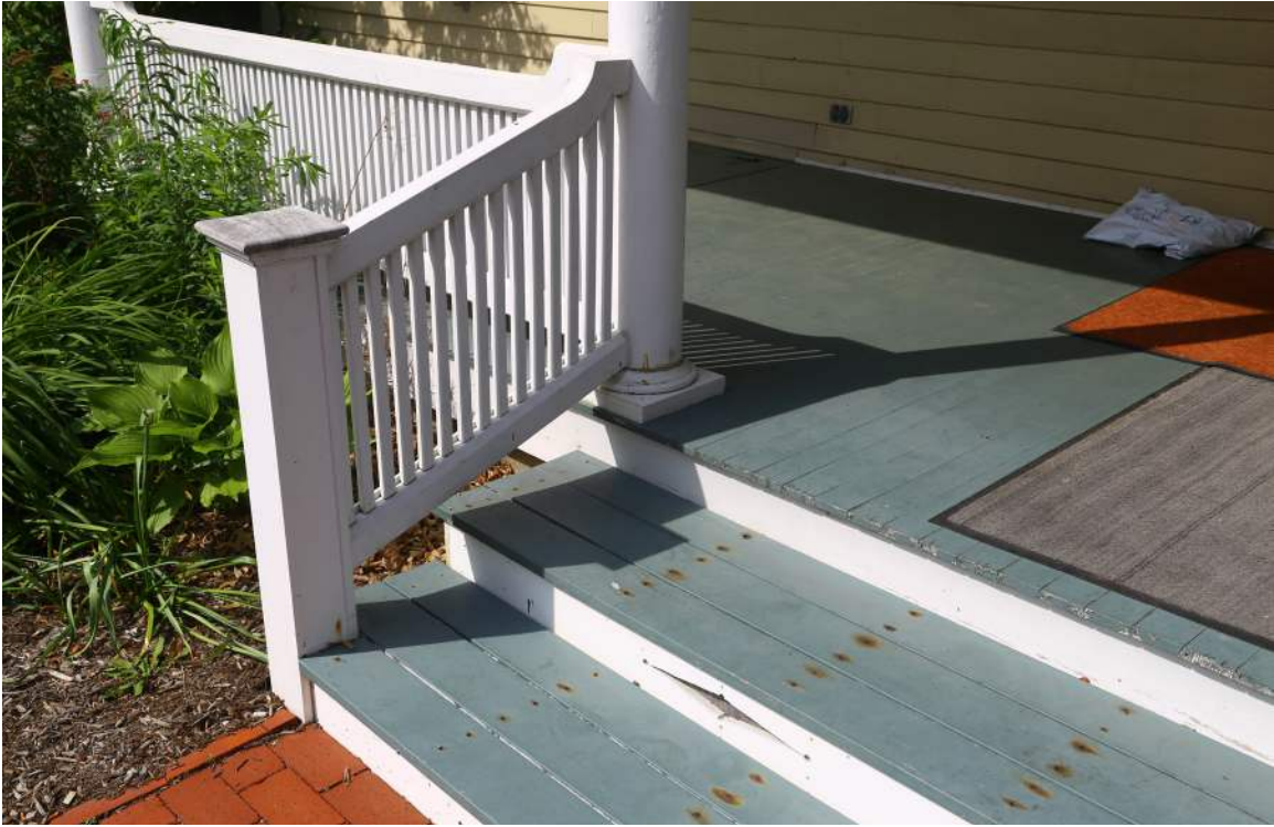
Figure 104. Representative area of the west porch showing typical paint issues, including failing paint at the nosing of the decking, rust stains at nail heads on stair treads, bare wood exposed on caps of newels, and caulking/epoxy repairs left unpainted (below).
