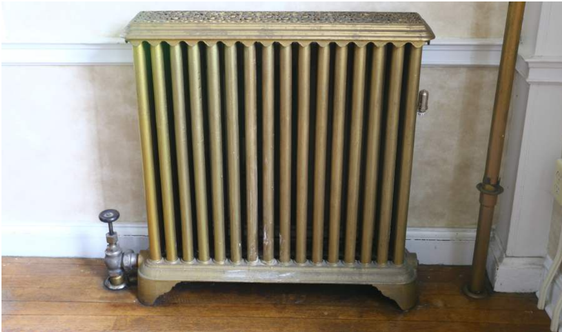
Figure 126. Some of the earliest steam radiators in the house are believed to be these column style cast iron radiators. The decorative casting that forms the top of the radiator simply sits on the columns. If this was removed, you would see that each column shaft is independent of the other. Each column screws into the base of the radiator and is closed at its top.
