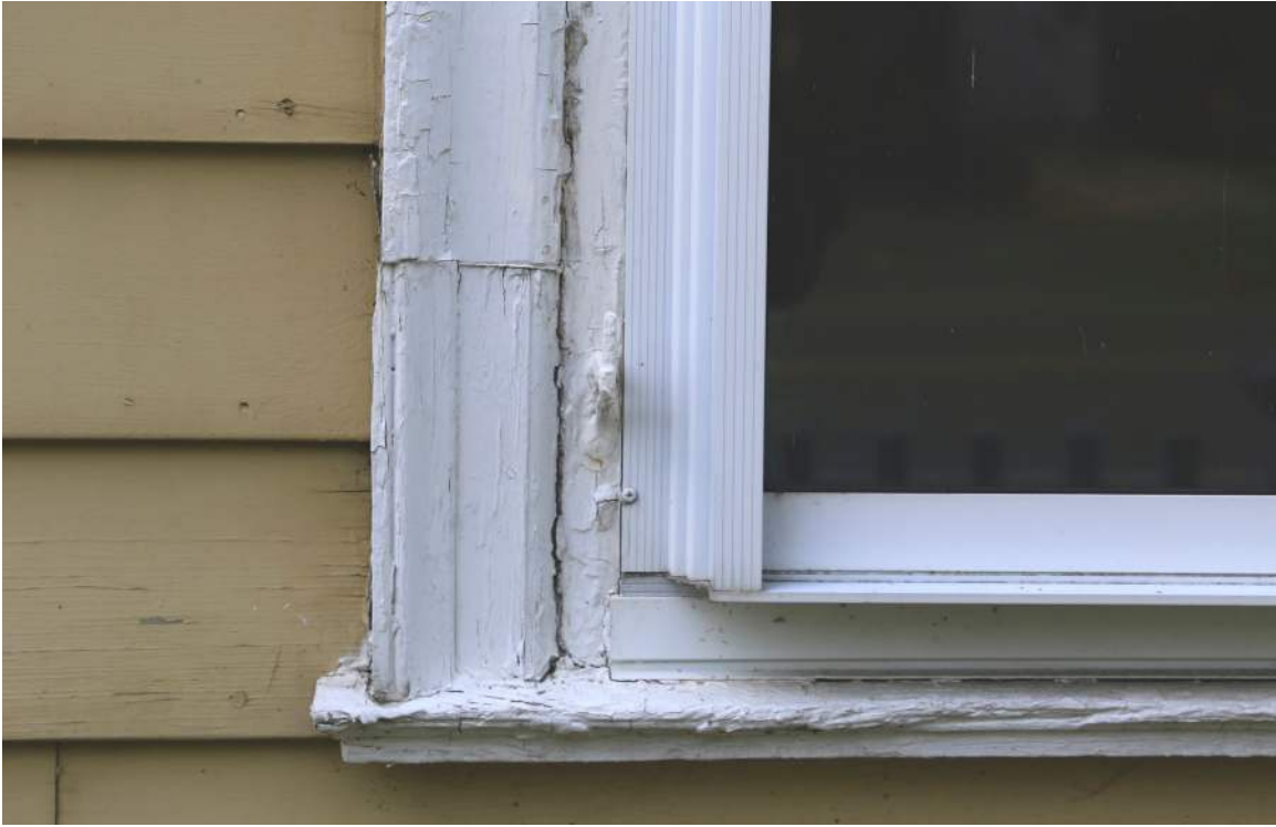
Figure 98. The window frames and other woodwork will likely need isolated repairs to deteriorated areas of woodwork and to correct past repairs where necessary.
