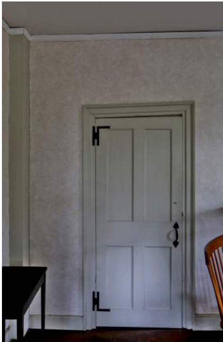
Figure 111. Room 202, Parlor Chamber, west closet door. The top of the door opening slopes down on the left side, towards the passage.
