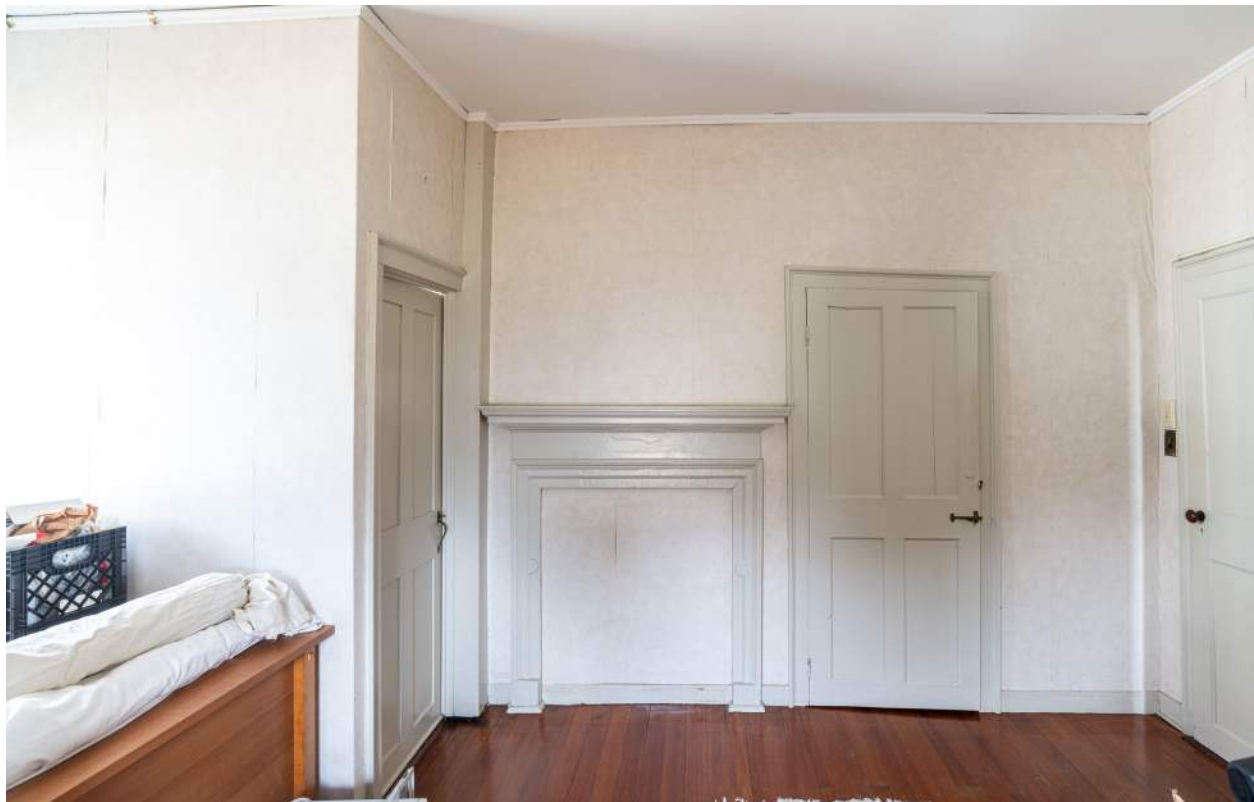
Figure 74. Shepherd House, right rear chamber (204). Note encroachment by bathroom at left.
