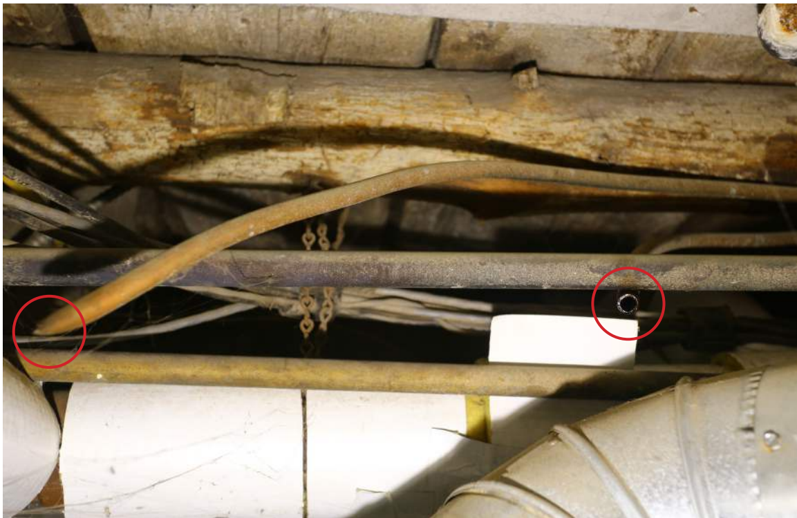
Figure 128. Cellar, west end above boiler. The red circles indicate the cut off ends of fuel lines from a previous fuel oil tank. The lines run to under the lean-to and exit the building underground to the west. These have every indication of serving a buried fuel oil tank. It is unclear if the tank has been removed or if it still remains buried under the yard or drive.
