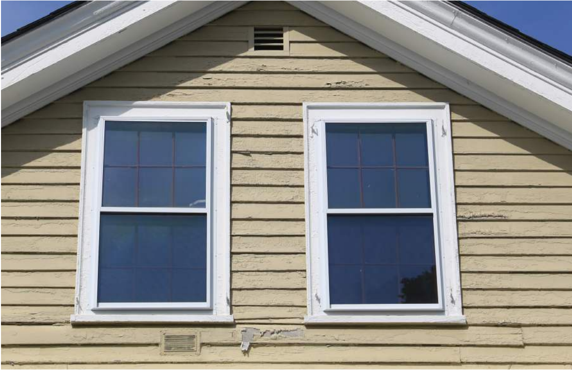
Figure 102. Detail of the west gable showing deteriorated and failing paint finishes on the clapboard siding.
