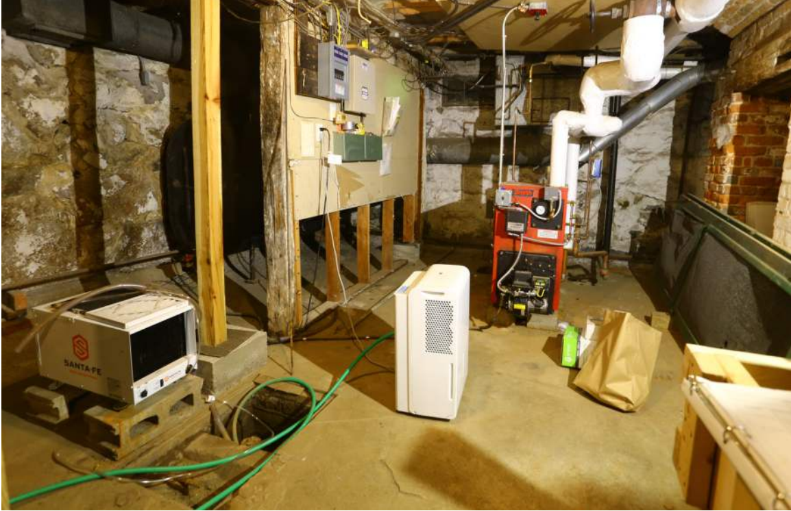
Figure 125. Cellar. The boiler and related components of the heating system are located in the southwest portion of the cellar. The fuel oil tank is visible behind the partition to the left of the image.
