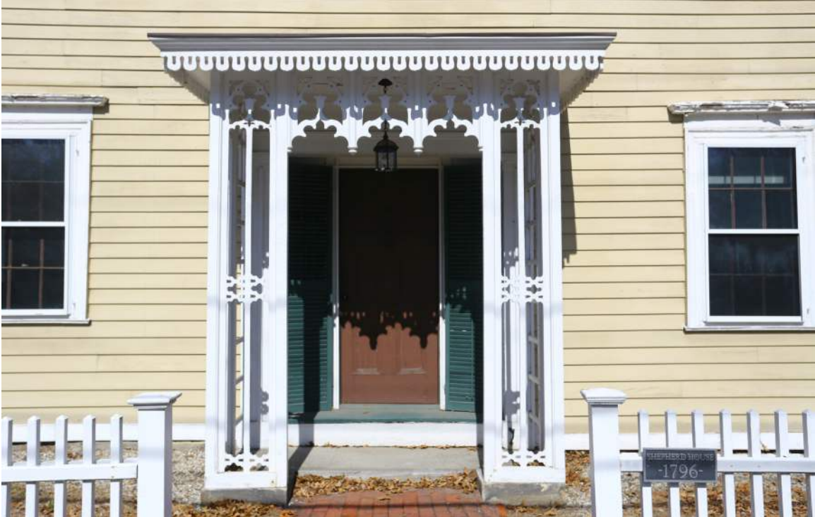
Figure 99. The south entry and portico are in good condition and only need minor repairs and repainting as shown in the following photographs. Note the failing paint on the window caps.
