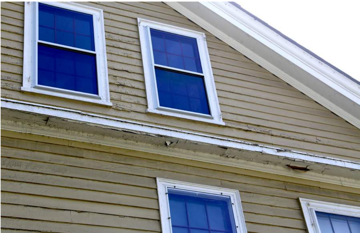
Figure 103. Detail of the east gable showing failing paint finishes on the clapboard siding and horizontal cornice.
