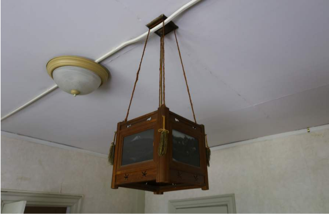
Figure 132. Room 202. This fixture showed power running to it with the light switch turned off when the wires and socket were probed with a voltage tester. All historic fixtures intended to be reused in the house must be inspected, updated and rewired to modern standards.
