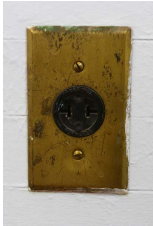
Figure 131. These early electrical outlets are not grounded and should no longer be used. In many cases, modern, surface mounted outlets have been installed adjacent to these.
