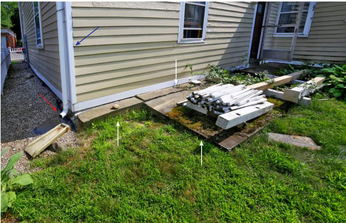
Figure 114. The concrete curbs and pads (white arrows) on the north side of the building should be removed. Ideally, leaders (red arrow) would tie into a subsurface drainage system connected to the municipal storm drains in the street to remove water from the perimeter of the building. The blue arrow identifies the location of the clapboards shown in the following image.
