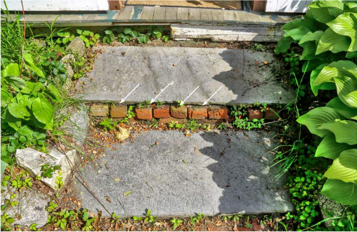
Figure 106. Steps to Lean-to. The bricks supporting the stone step are dry laid and have worked their way out from under the tread. They project out beyond the edge of the tread, posing a tripping hazard.
