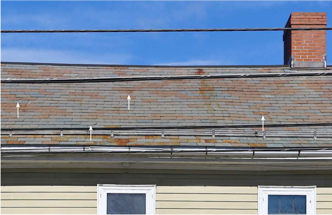
Figure 90. Detail of the south slope of the slate roof. The white arrows identify slates in this area that have broken corners, but are otherwise sound. The east chimney has an area of rotted brick at the attic level.
