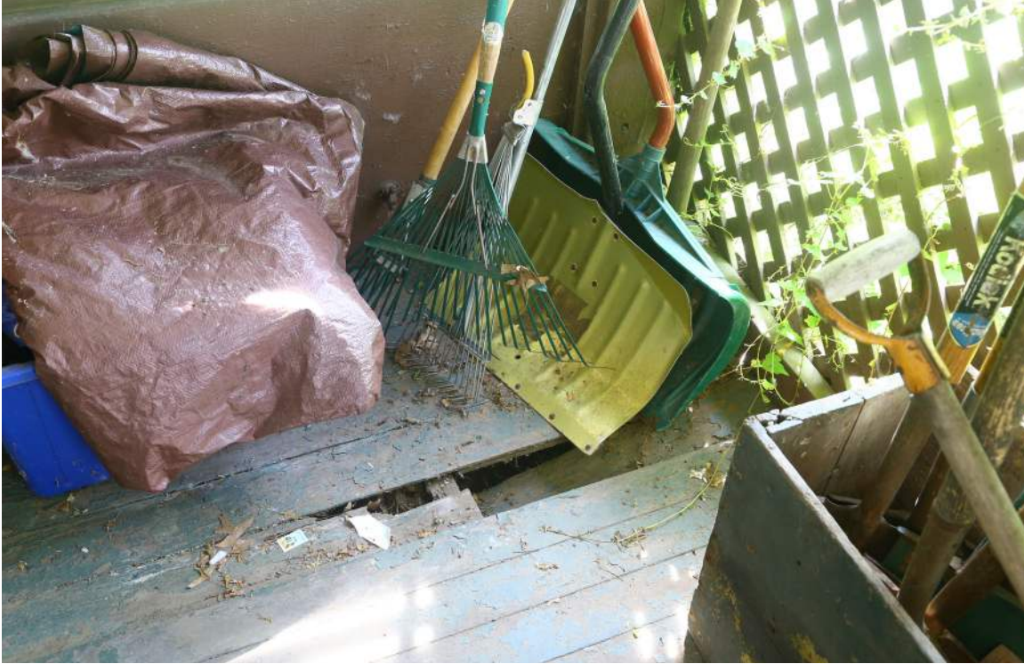
Figure 107. Rotted and broken flooring in the lean-to.
