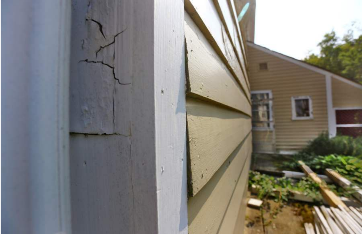
Figure 115. Northeast corner of the house, sighting towards the lean-to (west). A pronounced bulge in the north side of the wall is visible here. The butt ends of the clapboards (arrows) appear to have originally been installed flush with the face of the cornerboard. The bottom edge of the clapboards here are now approximately 1/4" proud of the cornerboard.
