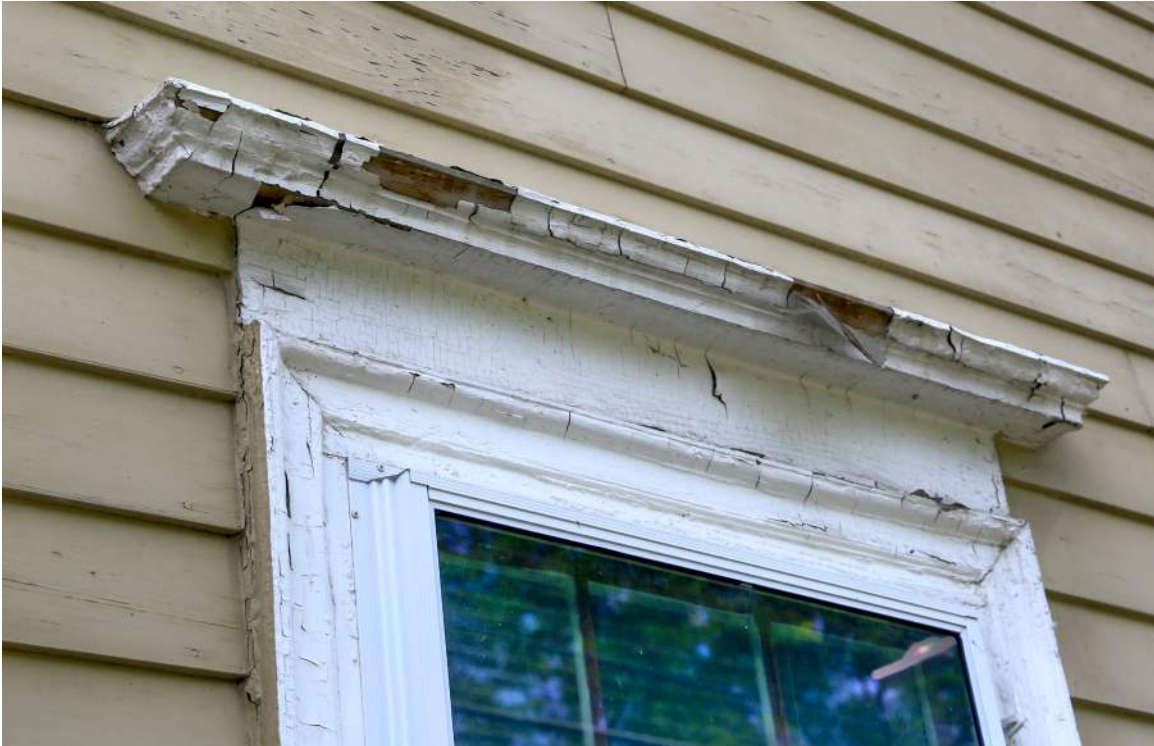
Figure 96. Representative example of failing paint finishes on the window frames. Original and early wood elements, such as the window frames and clapboards have heavy accumulations of paint buildup. This has reached a point where the surfaces no longer hold paint and are failing to bare wood.
