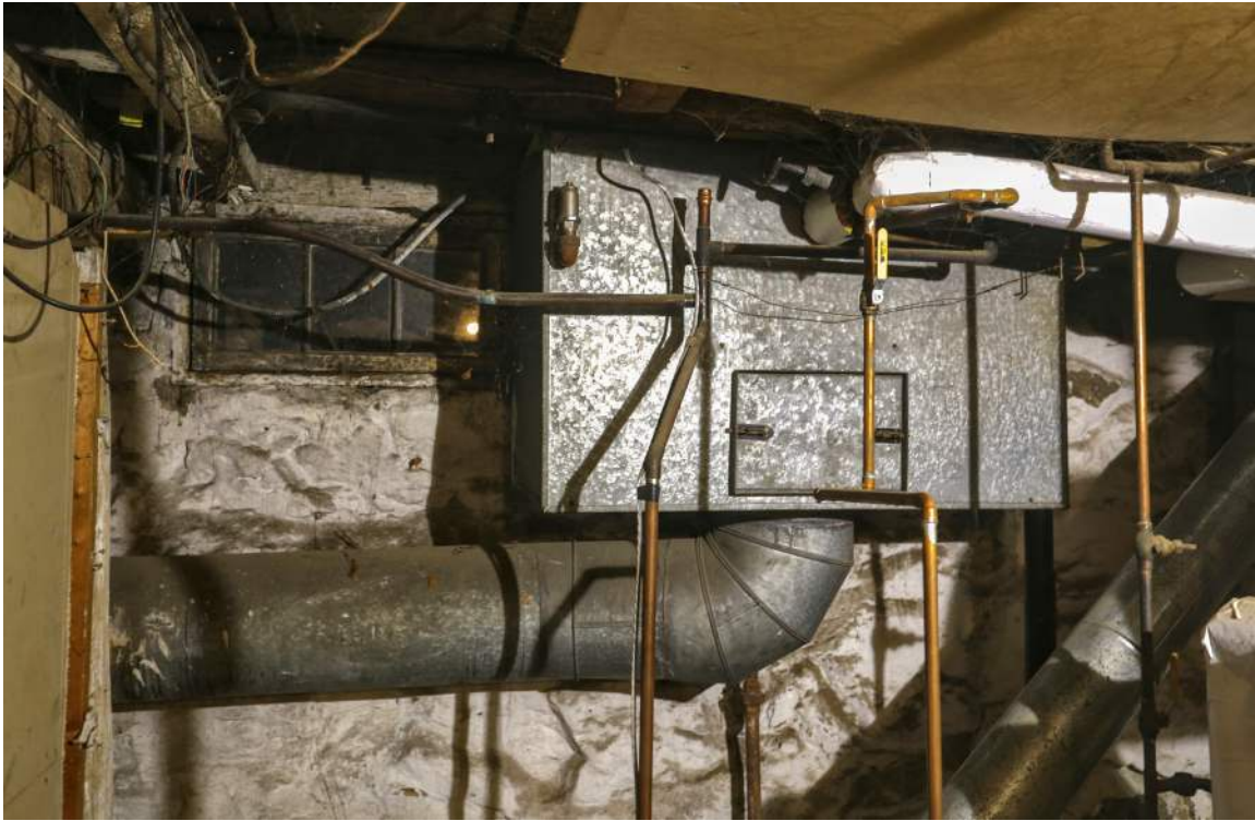
Figure 127. Cellar, west elevation. A ceiling mounted radiator box provides heat to Room 109. The box contains a radiator that warms air fed to it through the large duct entering from below. The duct is attached to the return air floor register on the south end of the room. This setup eliminates freestanding radiators within the room that take up floor space.
