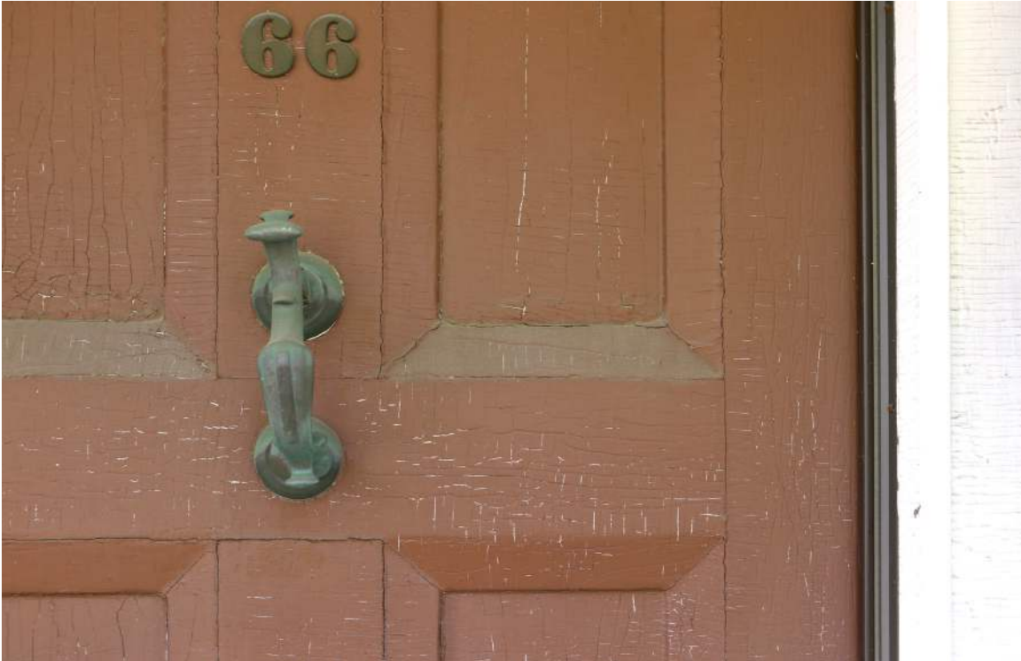
Figure 100. Detail of the south door showing crazing of the paint finish. The door retains good examples of hardware from the second quarter of the nineteenth century including the knocker, numbers and name plate (not shown).
