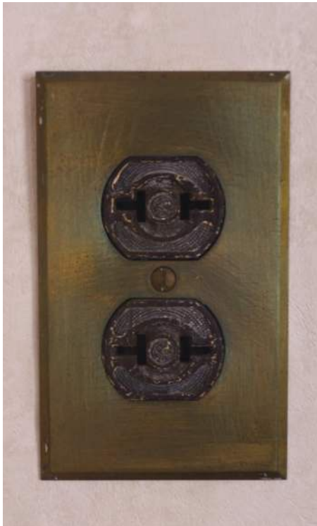
Figure 130. Early electrical outlets remain throughout the house, all of which, when tested were live and still providing power.
