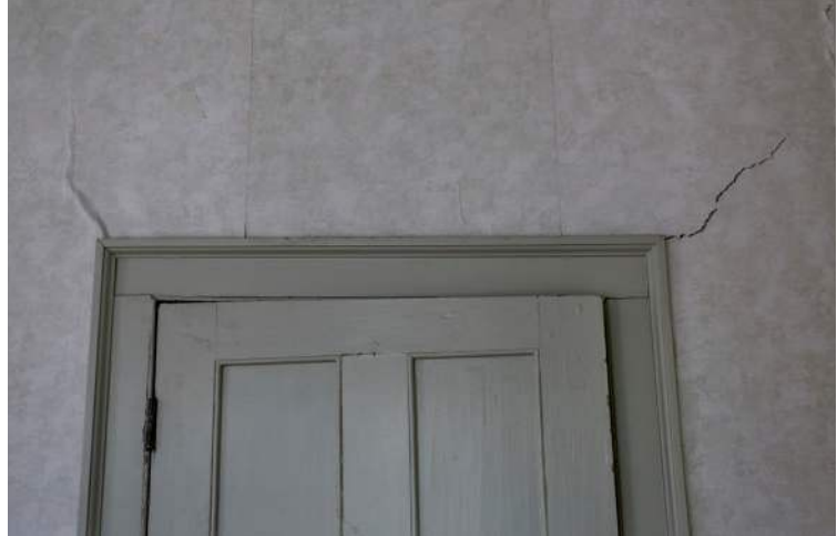
Figure 110. Detail of the top of the closet door opening in previous photo. The cracks in the plaster have occurred after the wallpaper was applied c. 2007 in preparation for Mass Humanities move into the building.
