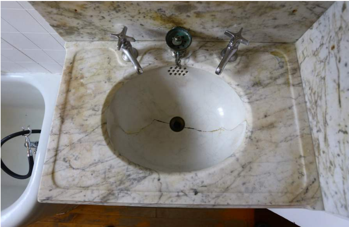
Figure 124. The sink in Room 206 is cracked. The crack has been repaired, but a small leak remains. A waste bin has been placed under the sink to capture any water dripping from the crack.
