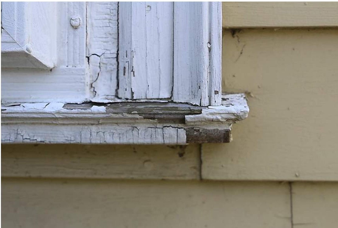
Figure 97. Detail of failing paint on exterior window sill. The window frames are original to the construction of the house and contain many fine molding profiles. Special care must be taken not to damage the molding profiles when the woodwork is prepped prior to painting
