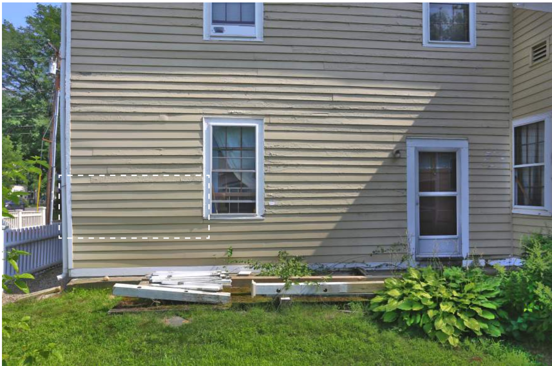
Figure 95. North elevation, east corner showing location of outward bulge found in the wall.
