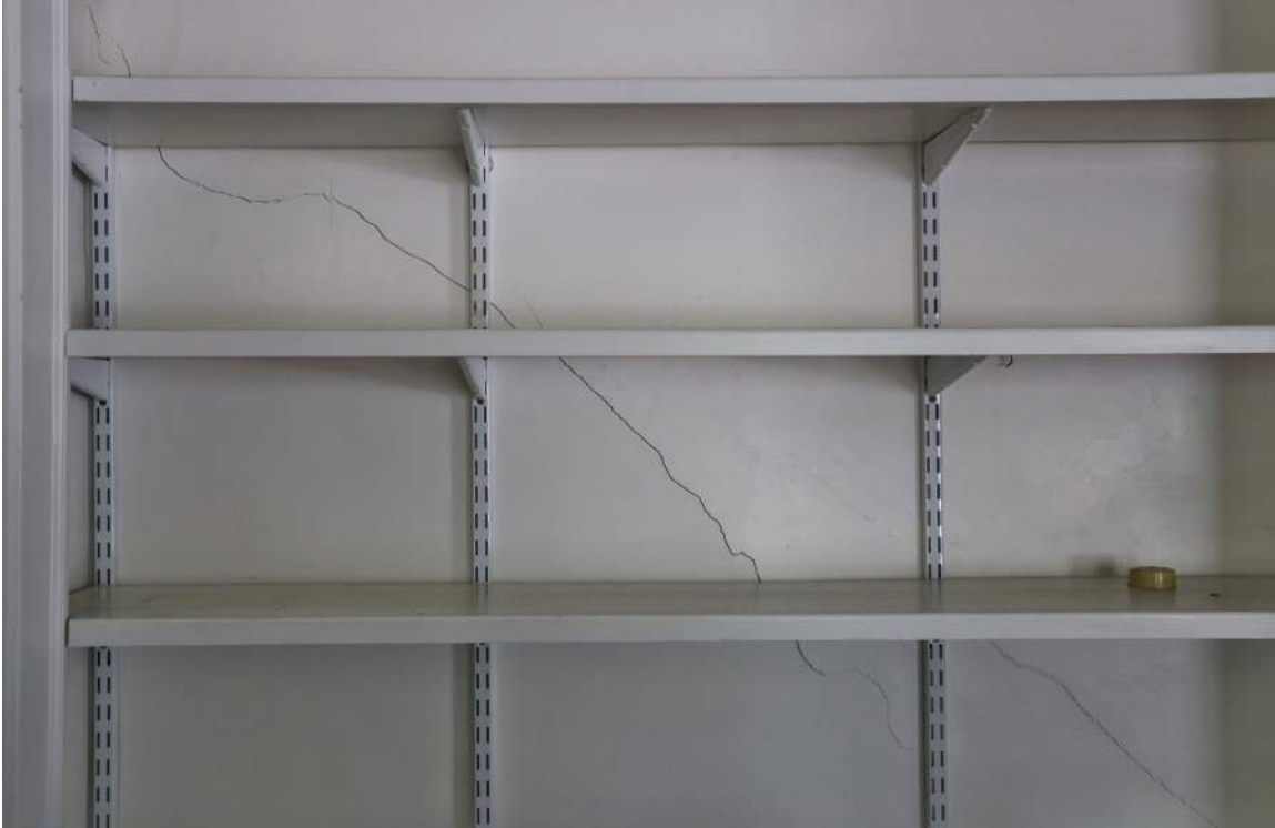
Figure 113. Room 102. North wall, west of the chimney. Settlement of the framing in the vicinity of the center passage, located opposite the left wall, has caused cracking in the plaster.
