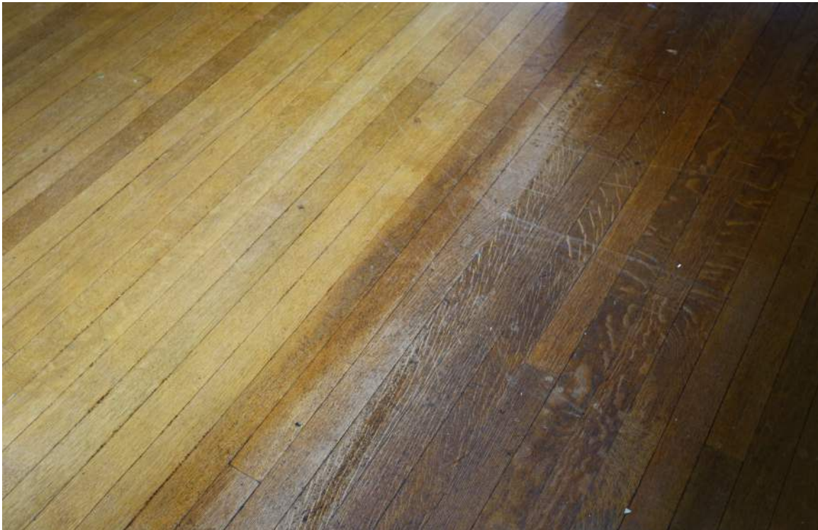
Figure 117. Flooring in Room 102 showing aged finishes. The lighter flooring was covered and protected from sunlight versus the darker areas around the perimeter of the room that were exposed.
