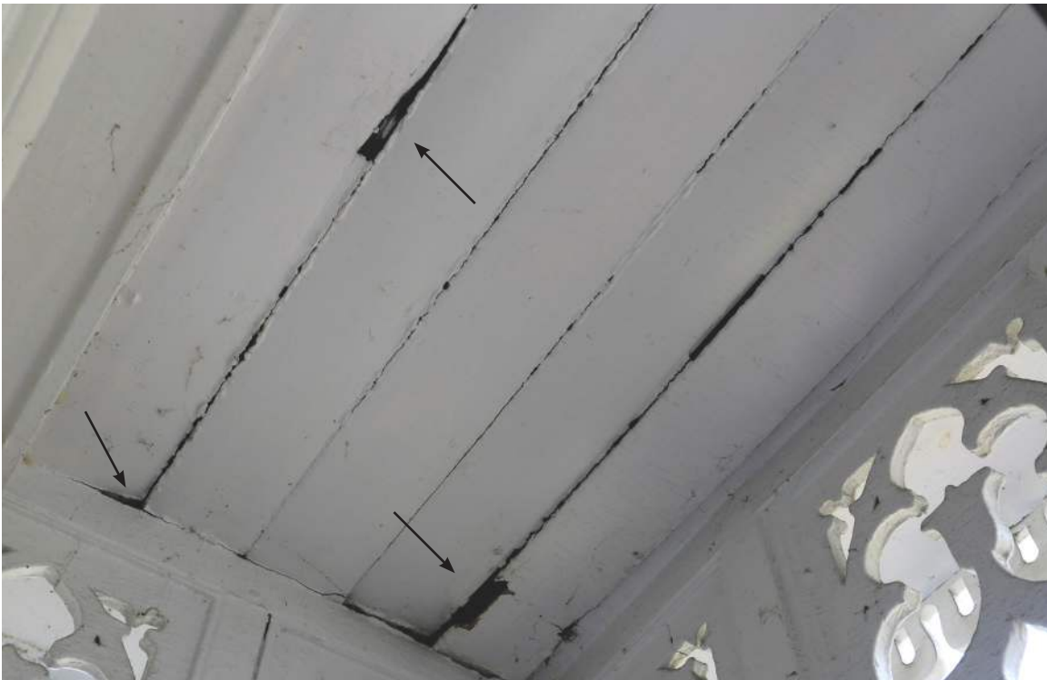
Figure 101. Cracks and openings in the board ceiling should be filled and patched to prevent insects and vermin from entering/ nesting in spaces within the building.
