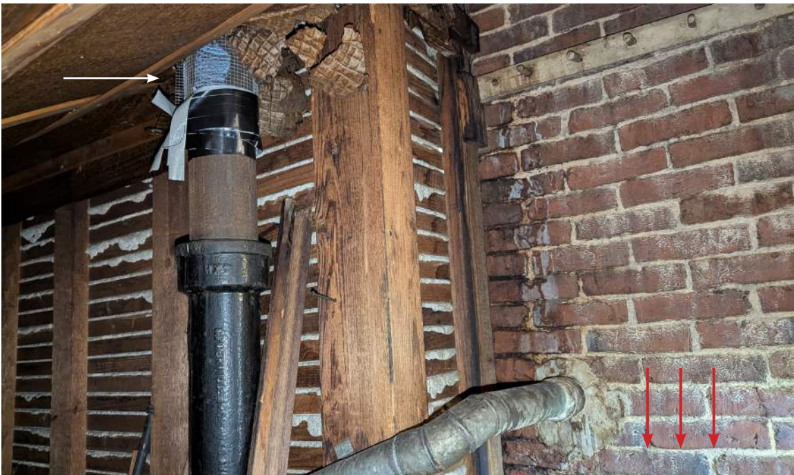
Figure 122. Attic, northeast room. A portion of the soil pipe is damaged and missing where it passes through the roof (white arrow). Not visible, but in this location, a portion of brickwork has deteriorated, creating a hole in the chimney (failures are in the direction of the red arrows). Daylight is visible in the hole, along with additional rotted brick dividing the flues.
